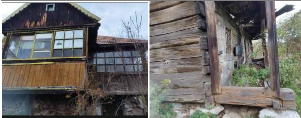
Fig.1 Abandoned rural dwelling illustrating advanced structural decay
